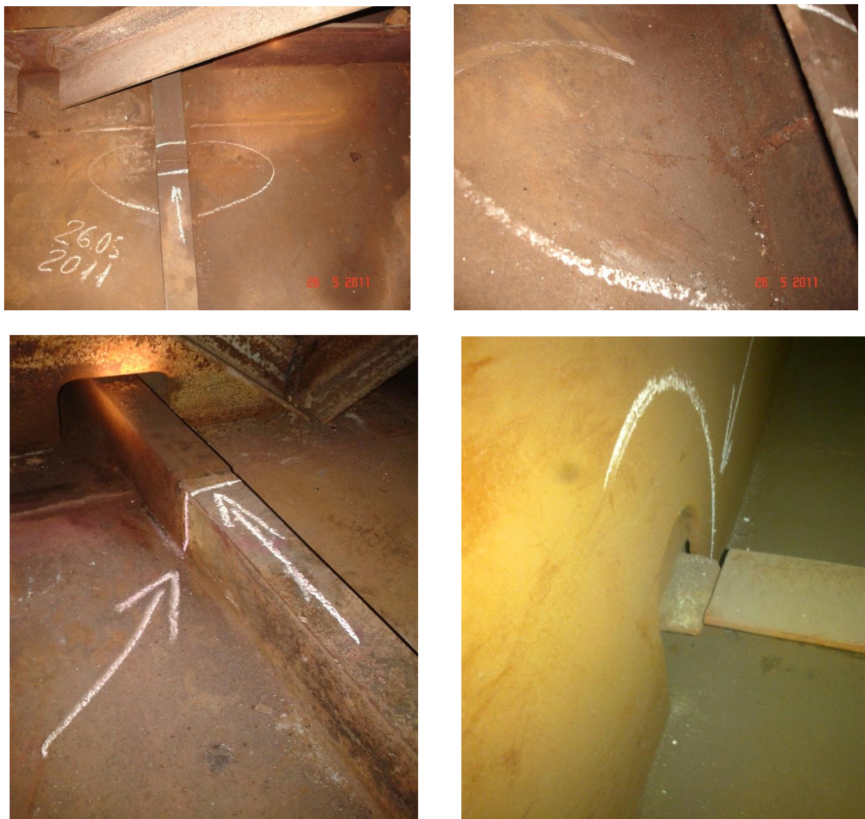
Fig. 6. Defects of the bottom boom of main beams
